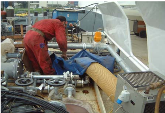
A PHE 25 heat exchanger creating heat & positive pressure
