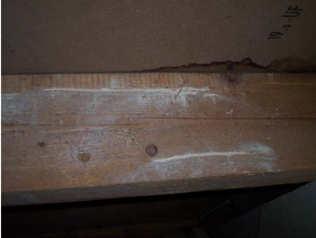
Figure 2, looking at a roof truss in the loft, shows a rare example of the larvae tunnel when it breaks through the surface. These two tracks are nearly 5mm in diameter.
