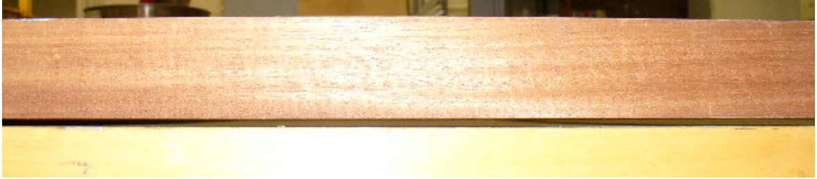
Figure 13: Hardwood external door - distortion 6mm over 1800 mm, after drying
