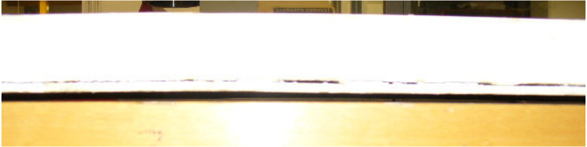
Figure 14: Internal pine door - distortion 12 mm over 1800 mm, and delamination of painted hardboard facing after drying
