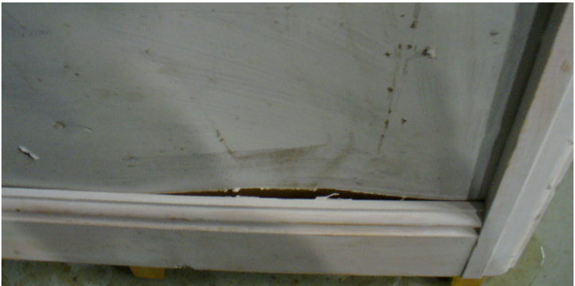
Figure 15: Plaster board panel - distortion after water saturation
